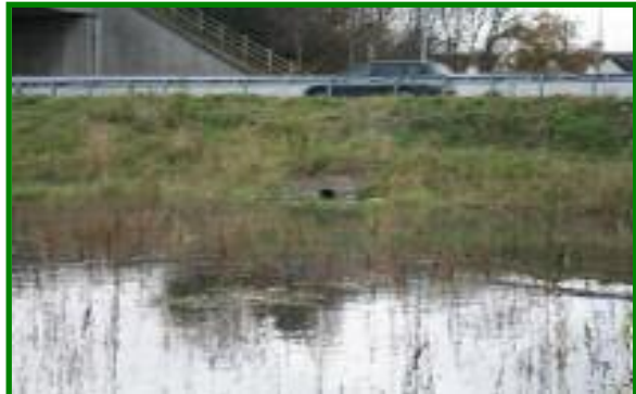
Fig 1: SUDS by Highway
